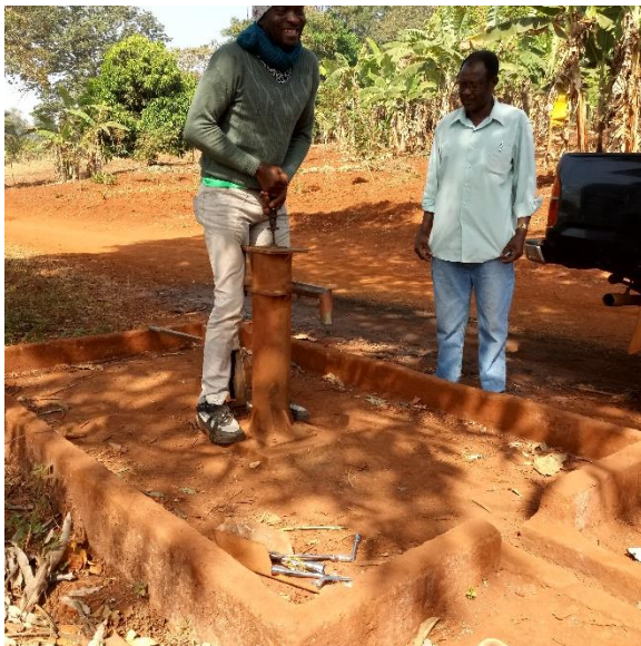
Testing if the cylinder is connected
