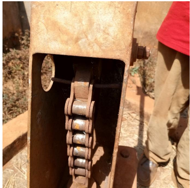
The pumping chain tied with nails instead of screws(boles)
