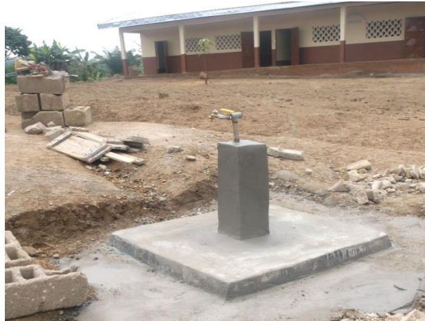
School portable water in EP Ngokop
